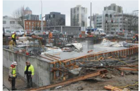
Workers have started pouring foundations and support for the $87.8 million College Station dorm being constructed for Portland State University. (Dan Carter/DJC)
