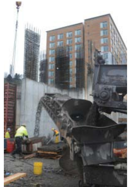
Workers must carefully place rebar, concrete and other materials as they construct the Portland State University College Station dorm building in the block between Southwest Fifth and Sixth Avenues and College and Jackson streets. (Photo by Dan Carter/DJC)
